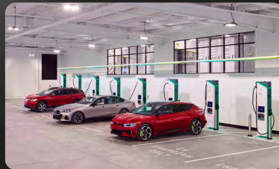
20 CHARGERS Downtown building lease, San Francisco, CA
