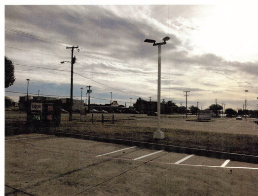
EXISTING POWER POLE, ELECTRIC METER AND LIGHT ARE REMOVED FROM THE SW SIDE OF PROPERTY.
