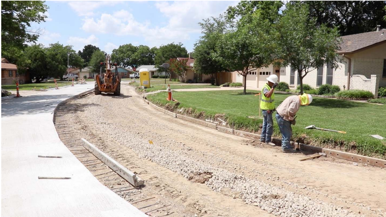
NRH Public Works street division crews replace a section along a residential street. In 2018, the Street Division resurfaced approximately 7.13 miles of residential streets. Additionally, the Street Division excavated and patched over 93,310 square feet of asphalt pavement; made around 7,651 square feet of concrete curb and gutter repairs; and patched a little over 4,800 square feet of potholes.
