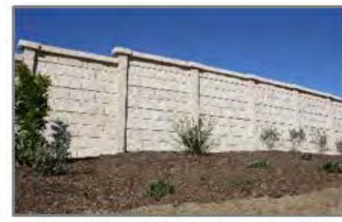
MASONRY WALL ON SOUTH PROPERTY LINE NEXT TO TARRANT COUNTY MAINTENANCE CENTER
